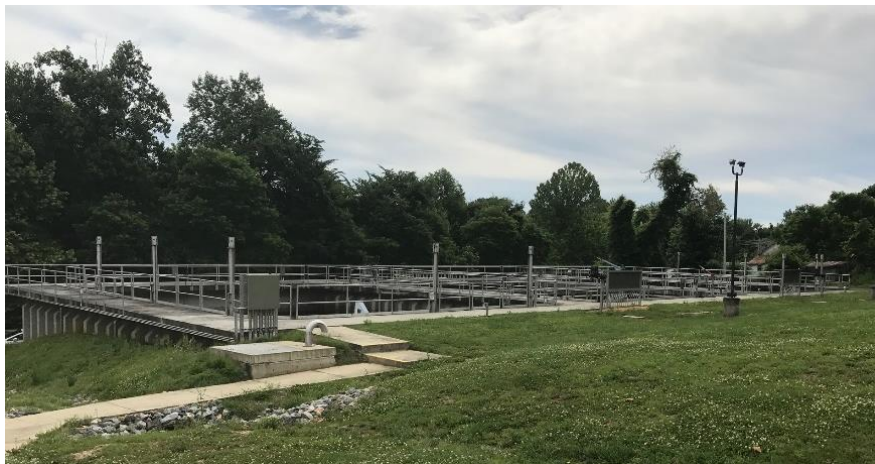
Figure 2.1: Centreville WWTP SBR
